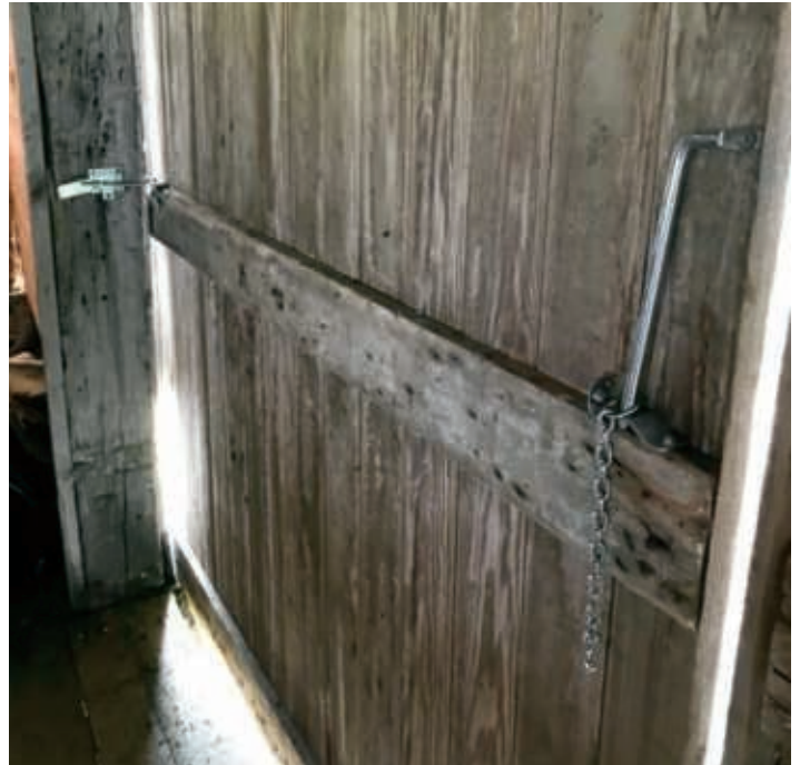
New hardware on the sliding barn door ensures they'll function properly and secure the main entryway from weather
