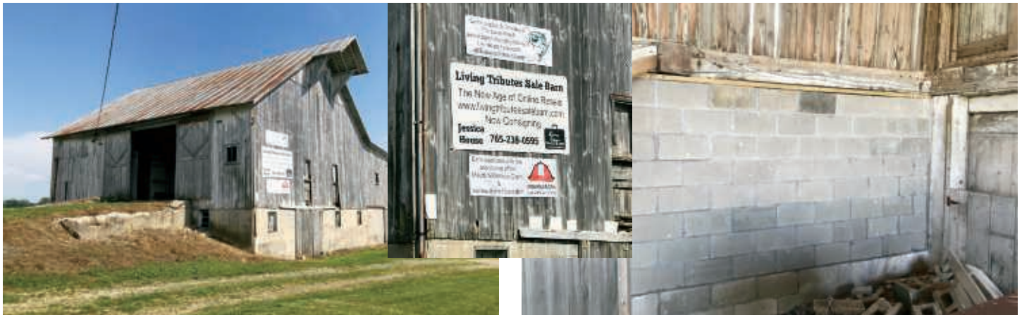
Jessica House's English bank barn, in Economy, Indiana, was awarded a grant from IBF in September of 2019. Some of her immediate needs were to repair a concrete wall of the dairy house that had collapsed and replace hardware on the barn door so the barn could be protected from weather.
