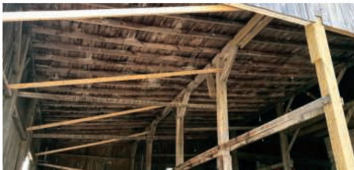
New support posts and a structural header were installed to rescue the integrity of the lean-to addition
